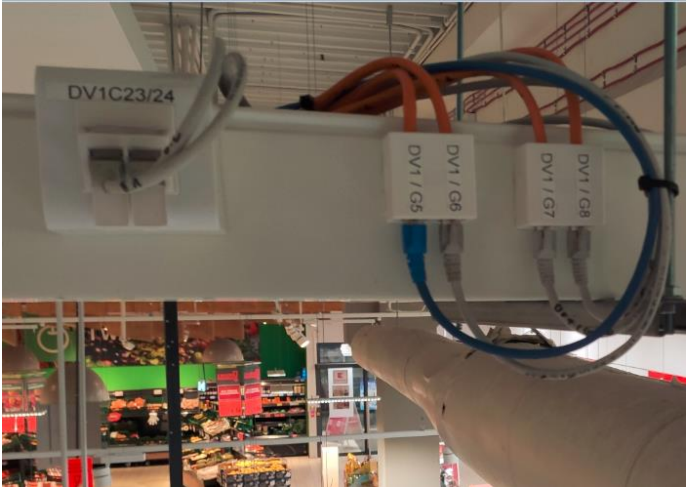
Standard Mini box Competition vs Mini Box Competition mounted on a cable tray
